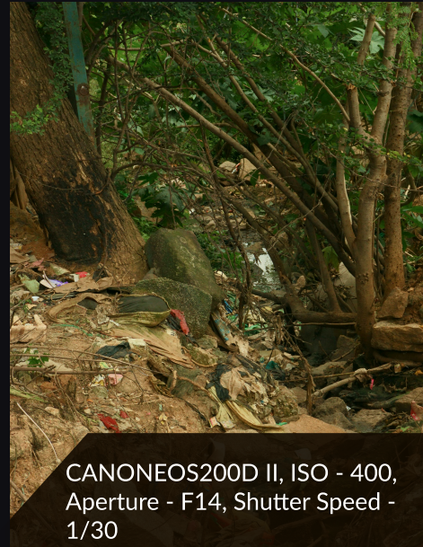
Litter clogs a parkside drainage channel.
