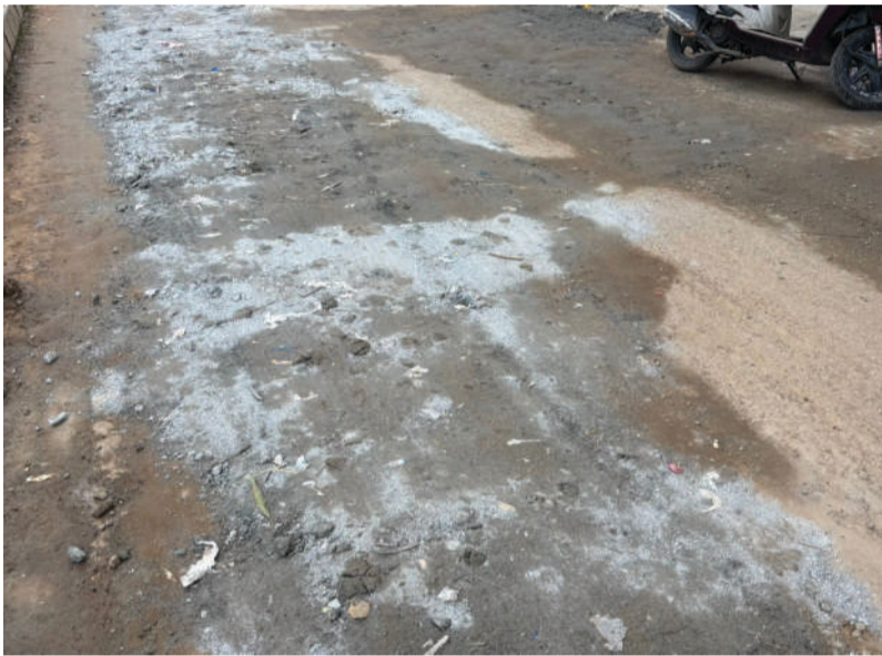
A residential street in Bengaluru shows signs of an unfinished and damaged patchwork after a failed repair attempt
