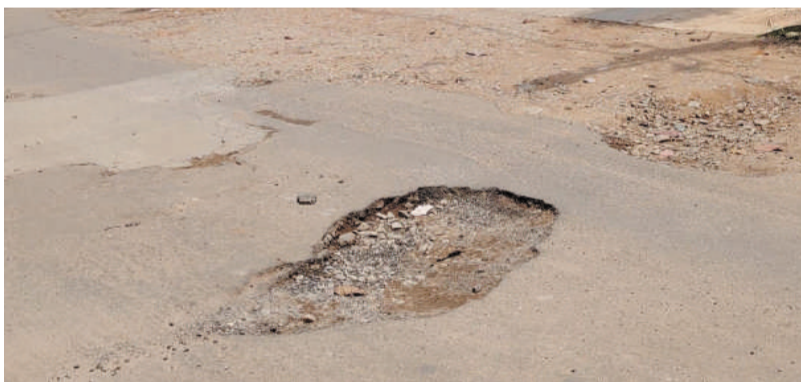
Potholes formed in road due to constant pipeline breakage
